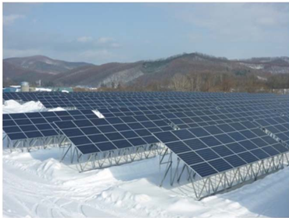
Ichigo Engaru Higashimachi ECO Power Plant (Hokkaido)
