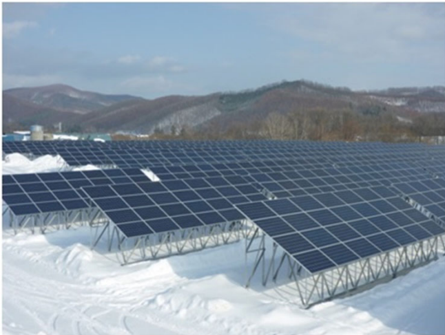
Ichigo Engaru Higashimachi ECO Power Plant (Hokkaido)
