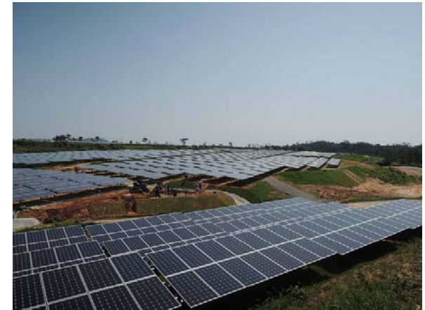
Ichigo Nago Futami ECO Power Plant (Okinawa)
