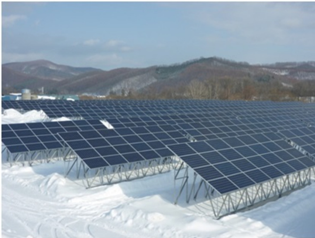
Ichigo Engaru Higashimachi ECO Power Plant (Hokkaido)
