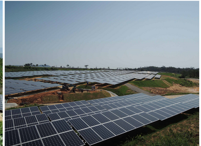
Ichigo Nago Futami ECO Power Plant (Okinawa)
