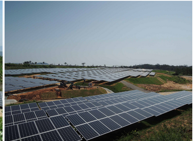
Ichigo Nago Futami ECO Power Plant (Okinawa)
