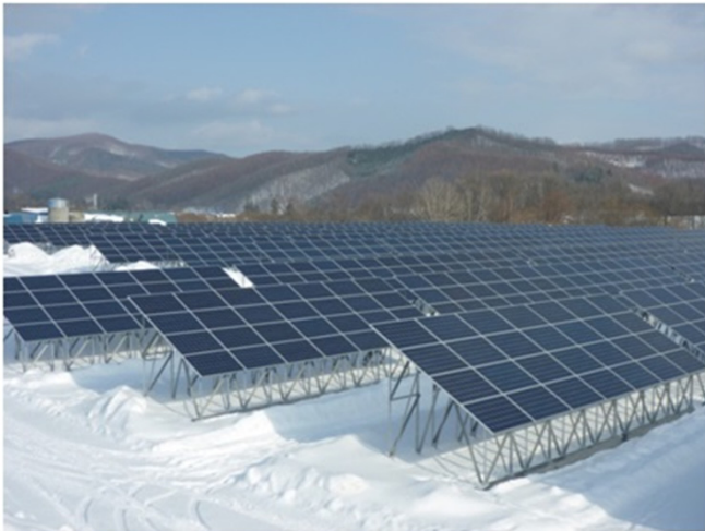
Ichigo Engaru Higashimachi ECO Power Plant (Hokkaido)
